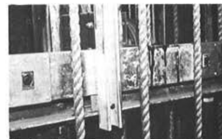
The fly gallery - ring intercom access points are available at no less than 64 different locations. Two can be seen in this picture.
