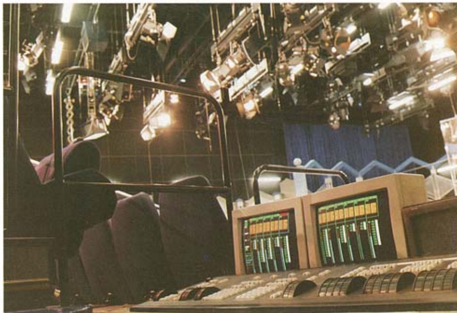
ADB S28 Series II control system at the Studio House.
