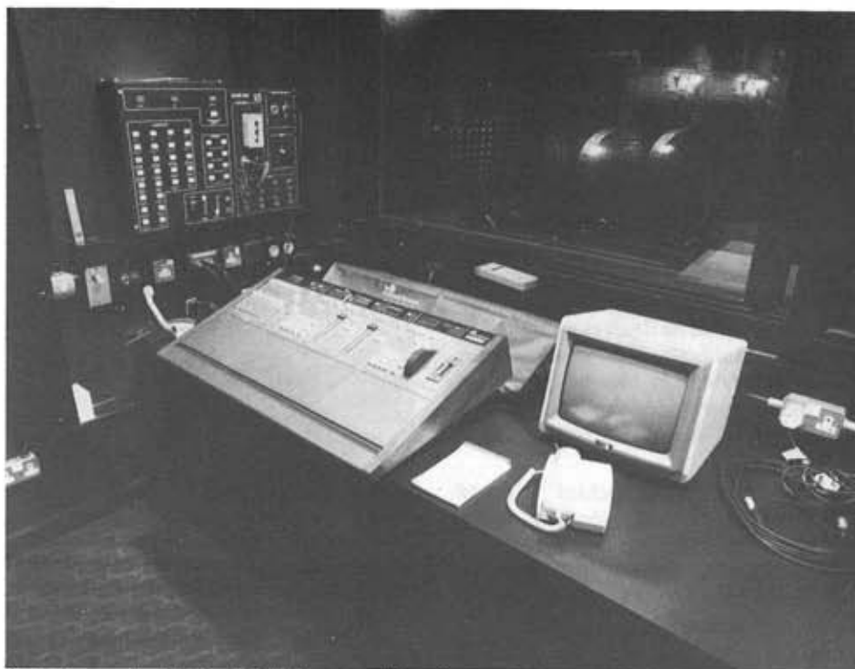
Control room showing Gemini lighting control board.
