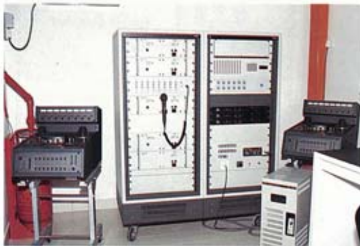
Control equipment racks with two Otari multi-track tape machines (duty and standby), UPS and halon gas cylinder.
