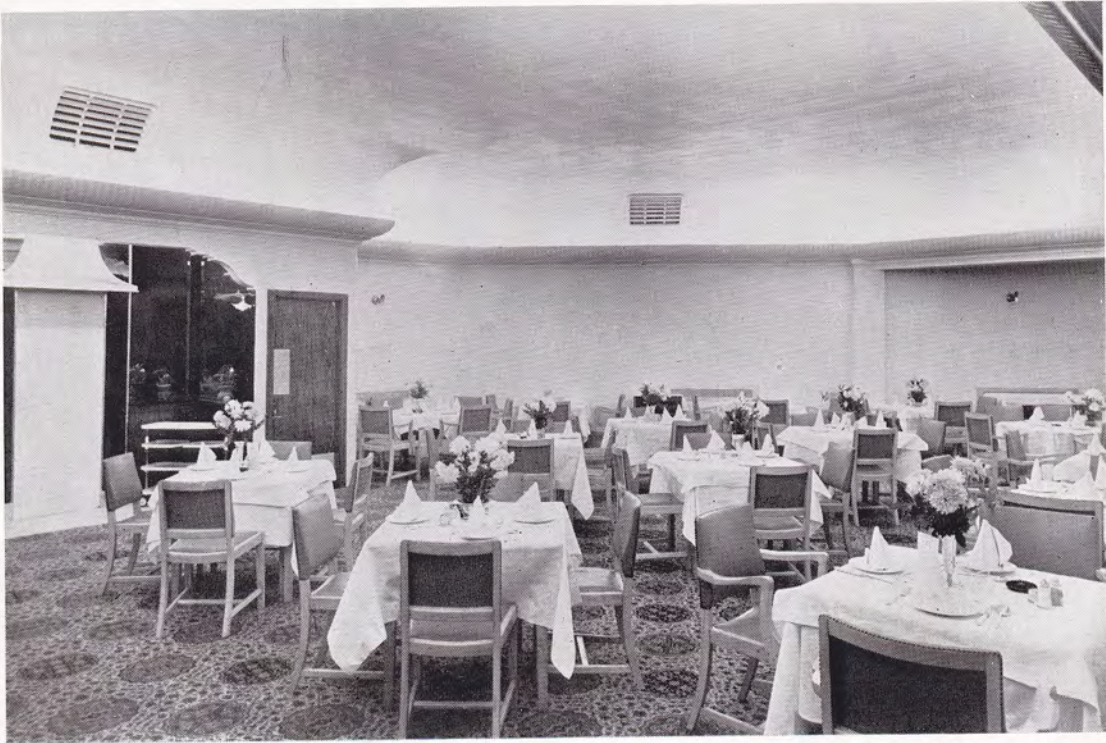
Indirect cold cathode lighting at the Clarendon Restaurant, Hammersmith.
