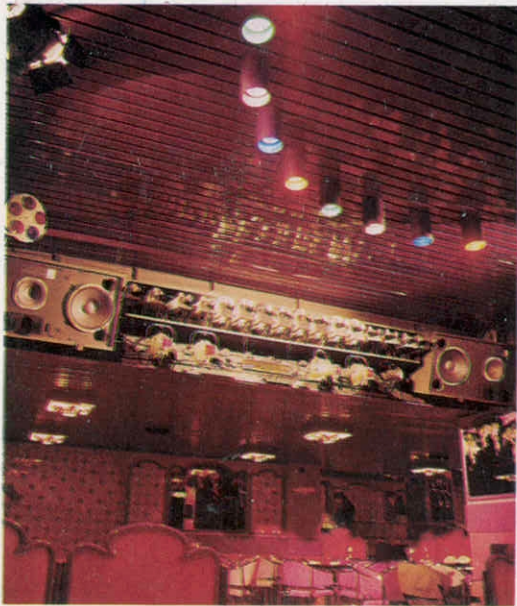
▲ Cindy's - Stockholm, Sweden: Installation by Juliana's Sound Services Limited.
