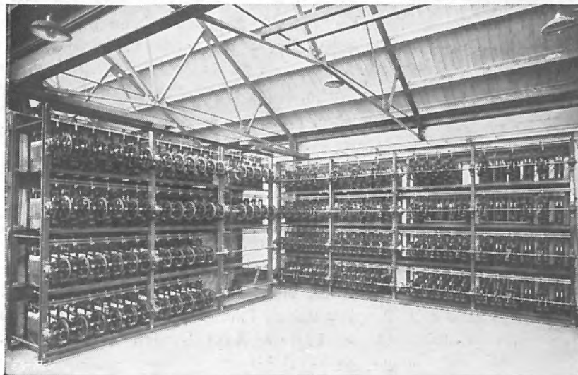
Covent Garden Opera House Dimmer Bank
