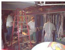
The main dimmer room installation
