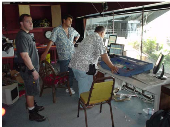
Joel Savoie looks on as Otto Alvarado of Strand Lighting and George Pasi use the control console to test the system
