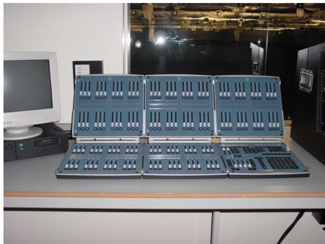
A 300 series desk and Outlook architectural controls were specified for the theatre
