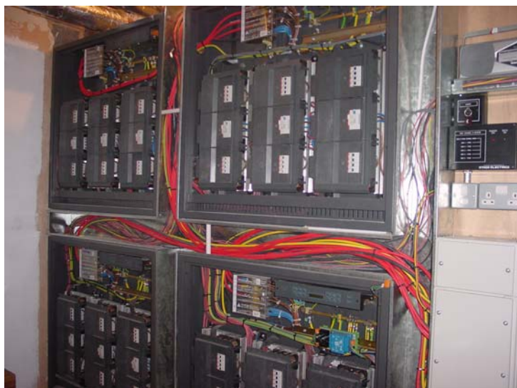
The LD 90 dimmer racks being installed by Stage Electrics
