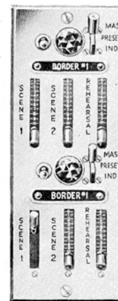
Figure 3. Typical Circuit Panel with two controls on one panel. Each has Two Scene Presets, and a Rehearsal Control, switch and pilot indicating light for circuit contactor, selector switch for direct independent control, color master control or preset control through Scene Masters.
