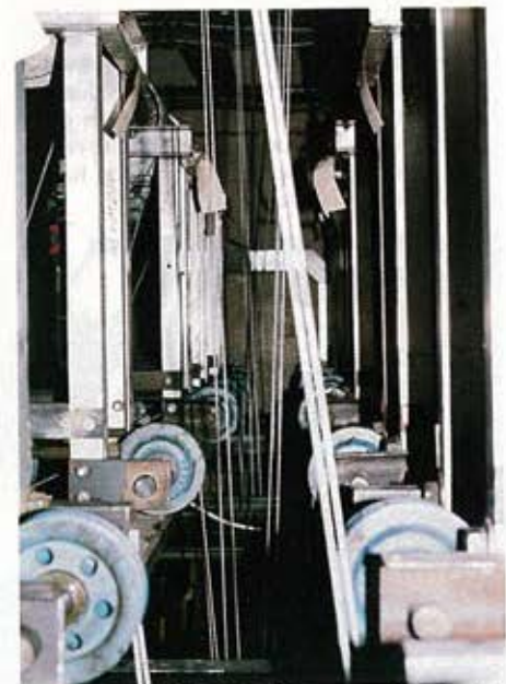
View on the fly floor between the double stacked rows of 23 winches.
